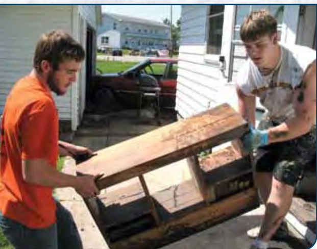
Two Wartburg College students carry furniture out of a flooded house
